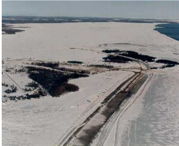
Fig. 11: Aerial picture to north of completed channel across McLaughlin Lagoon and work underway on Whalen Property
