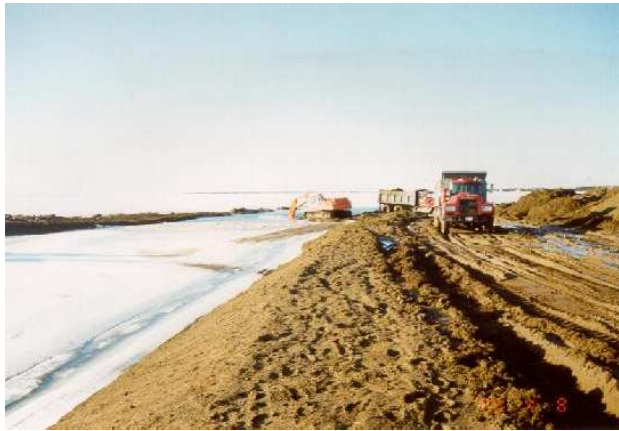
Fig. 8: Removal of “dredged” sediment by truck. Note opened channel to left of picture
