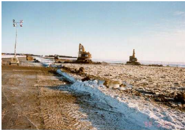
Fig. 9: Dredging in Little Tracadie Lagoon. Note temporary light standard to permit 24-hour operations.
